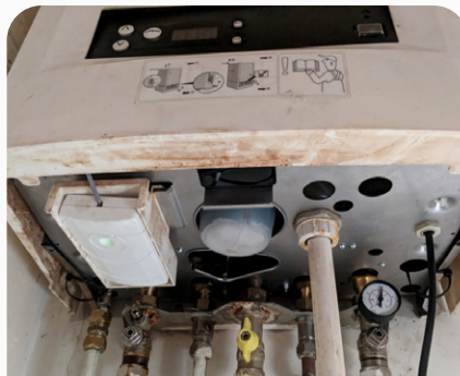
Issues relating to inadequate heating and hot water
