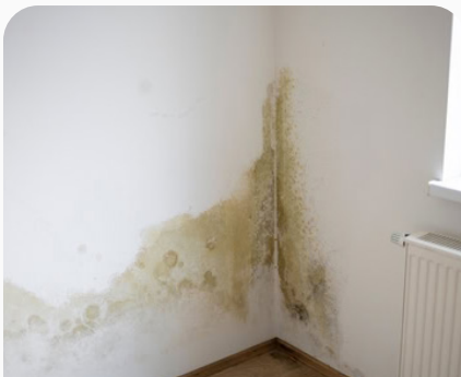
Damp and Mould
